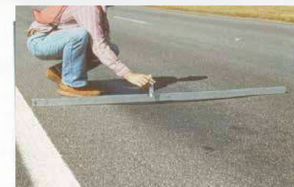
Figure 15a. Low-Severity Rutting.
