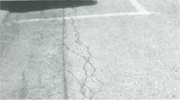
Figure 7b. Medium-Severity Edge Cracking.
