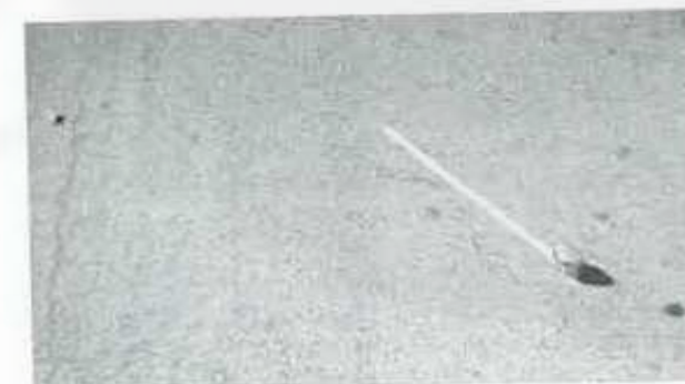
Figure 17a. Low-Severity Slippage Cracking.
