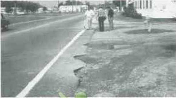
Figure 7c. High-Severity Edge Cracking.
