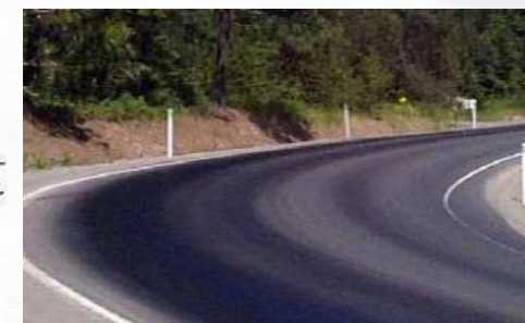
Figure 2b. Medium-Severity Bleeding.
