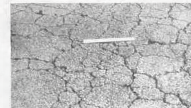
Figure 1c. High-Severity Alligator Cracking.
