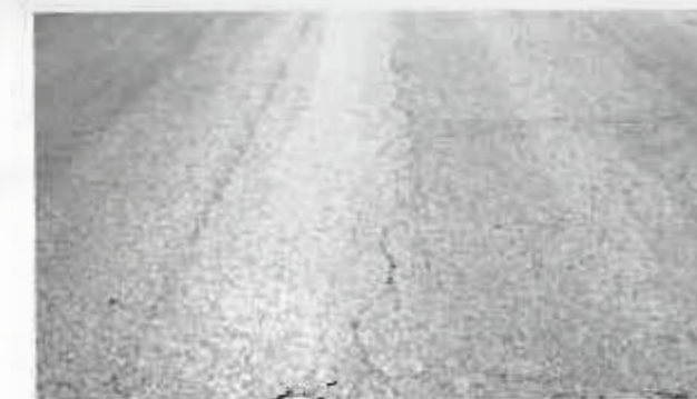
Figure 1a. Low-Severity Alligator Cracking.
