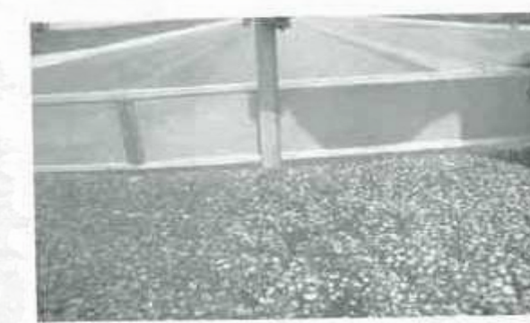
Figure 15b. Medium-Severity Rutting.
