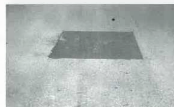
Figure 11a. Low-Severity Patching and Utility Cut Patching.
