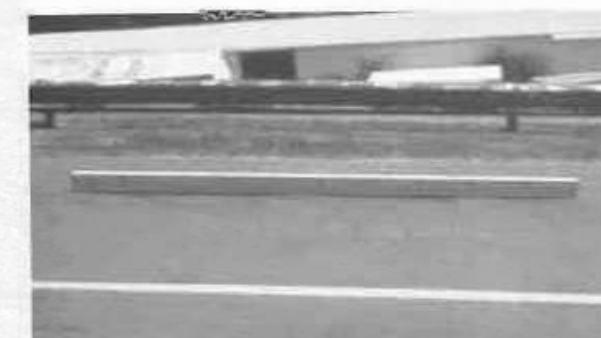
Figure 5b. Medium-Severity Corrugation.
