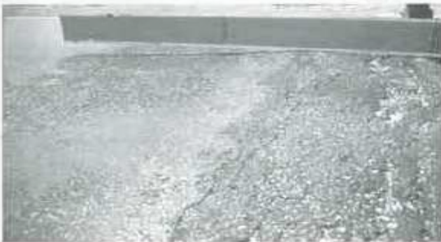
Figure 4c. High-Severity Bumps and Sags.
