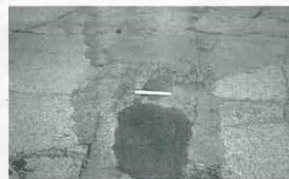
Figure 11c. High-Severity Patching and Utility Cut Patching.
