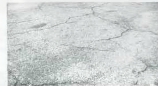
Figure 3a. Low-Severity Block Cracking.
