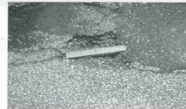
Figure 13a. Low-Severity Pothole.
