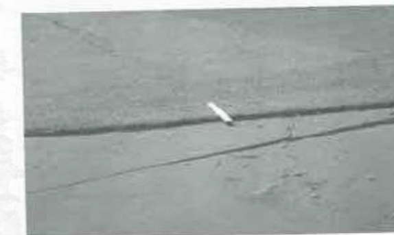
Figure 16b. Medium-Severity Shoving.
