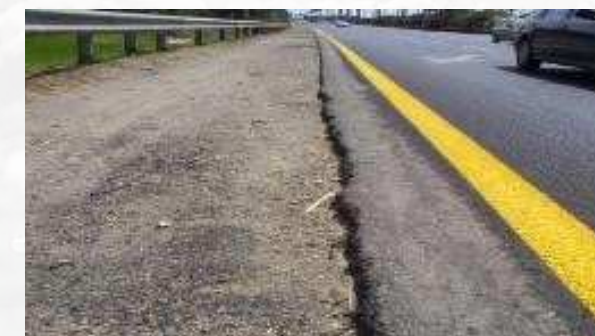
Figure 9c. High-Severity Lane/Shoulder Drop-Off.
