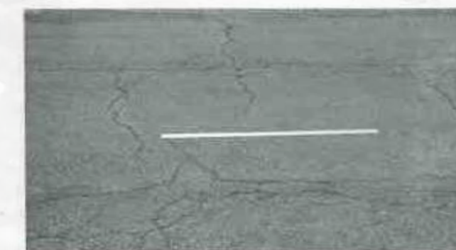
Figure 3c. High-Severity Block Cracking.
