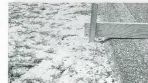
Figure 9a. Low-Severity Lane/Shoulder Drop-Off.
