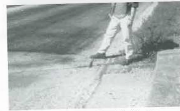
Figure 16a. Low-Severity Shoving.
