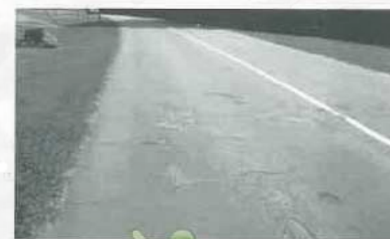
Figure 19c. High-Severity Weathering and Raveling.
