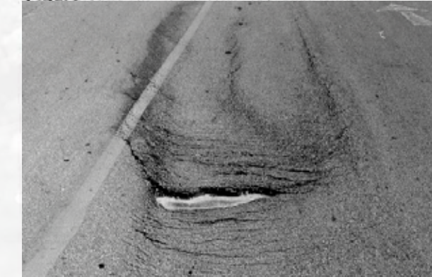
Figure 17c. High-Severity Slippage Cracking.
