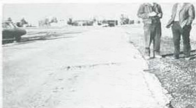
Figure 4b. Medium-Severity Bumps and Sags.
