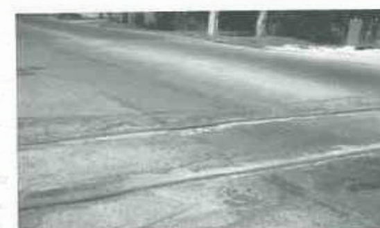
Figure 14b. Medium-Severity Railroad Crossing.
