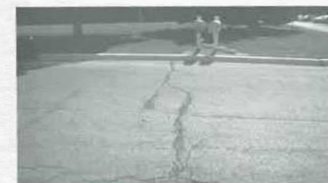
Figure 3b. Medium-Severity Block Cracking.
