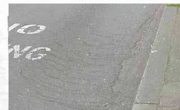
Figure 17b. Medium-Severity Slippage Cracking.
